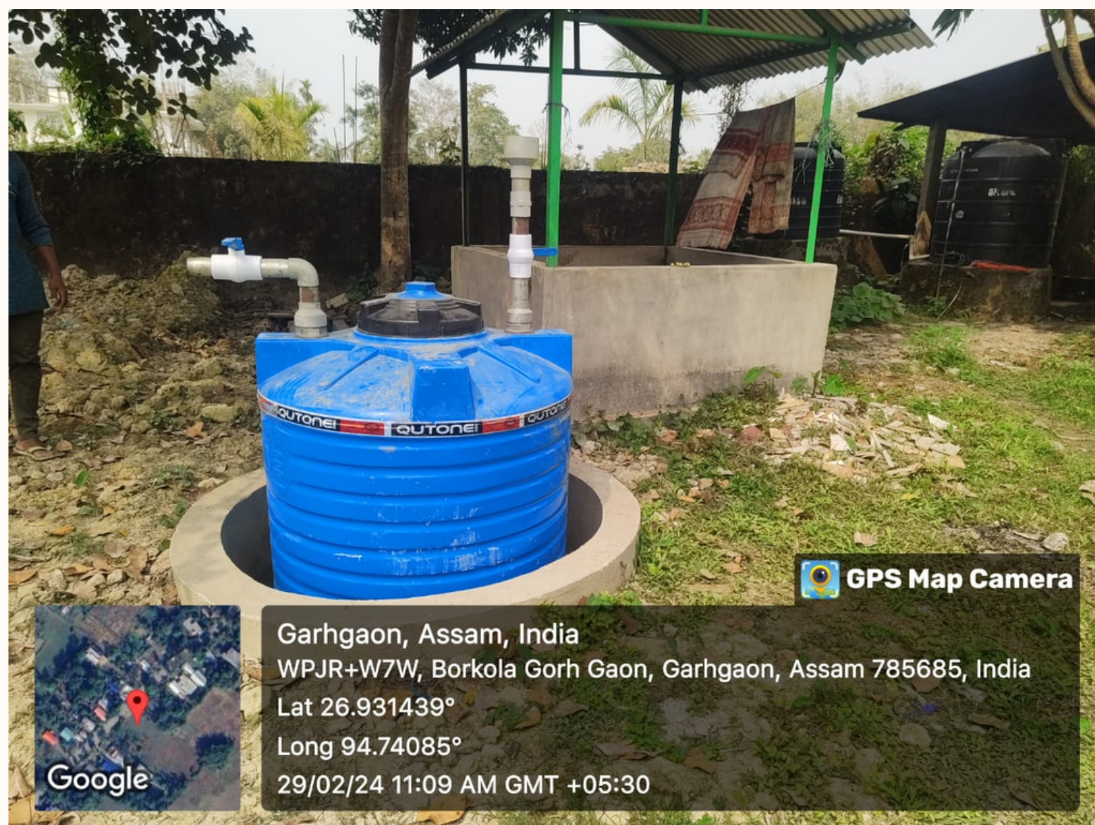
Picture: Biogas plant in campus
