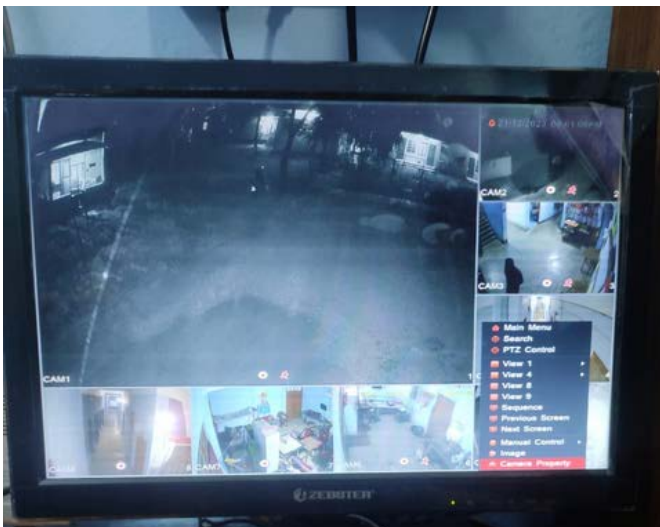
CCTV surveillance (Girls' Hostel)
