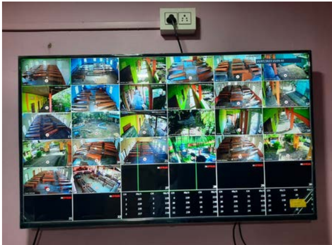
CCTV surveillance (College Campus)
