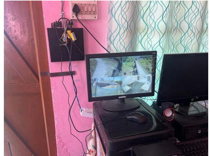
CCTV surveillance (Boys' Hostel)
