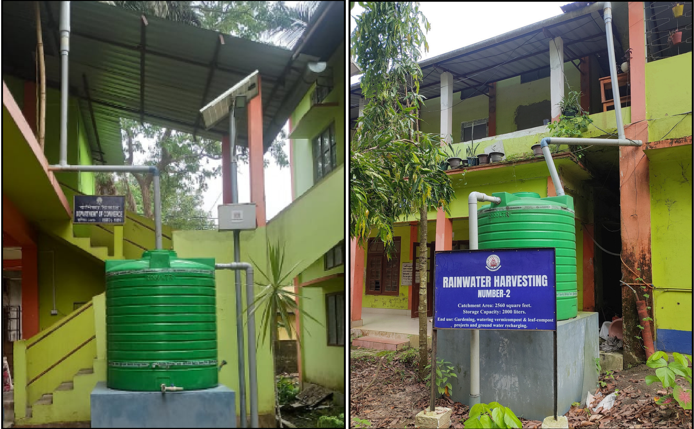
Rainwater harvesting tanks
