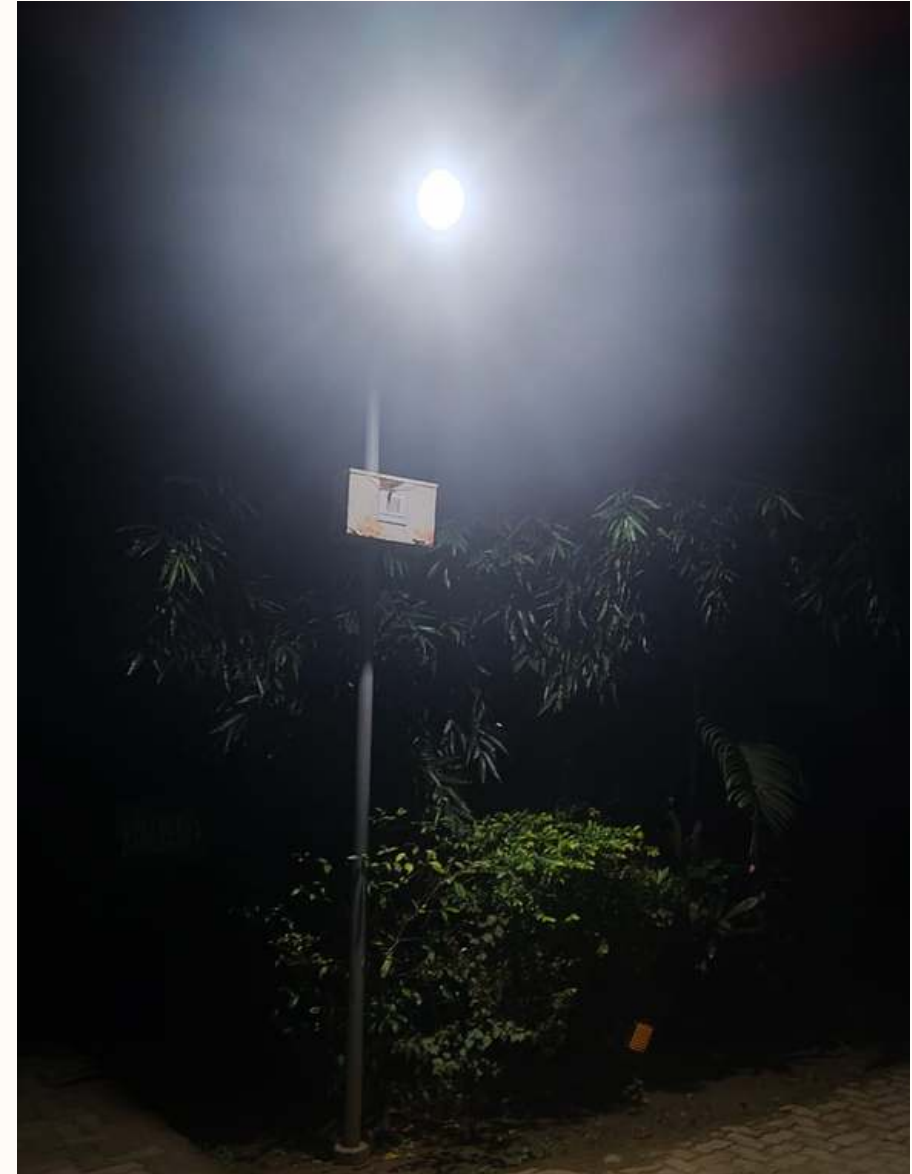
Solar Street lights
